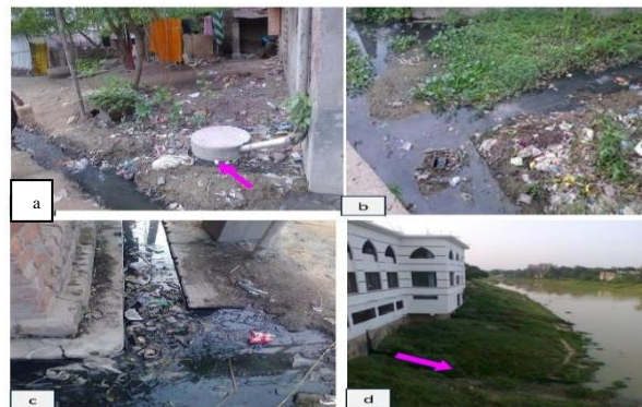
Fig. 4: Photograph Showing (A) the Drainage System at Kazirmore (the Arrow in the Photographs Indicate Sanitary Leaching Mixed in the Drainage System, (B,C) Household Wastes Fill the Drain That Is A Signature of Unconsciousness (D) Outlets of the Drain in the Choto Jamuna River Water (Arrow Sign Indicates Waste Water Mixing in the River).
