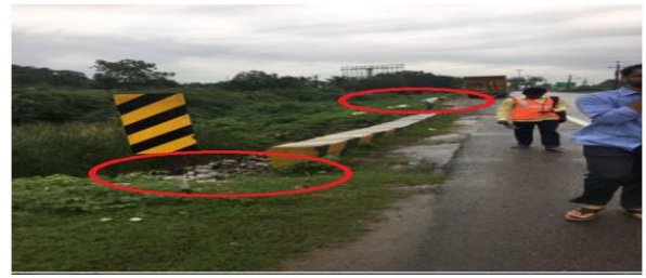
Fig.8: at chainage: 266.500km LCW.
