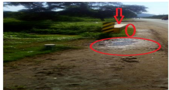
Fig.22: at chainage: 254.605km.LCW
