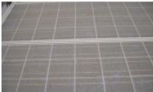
Fig. 3: Solar module covered by heavy layer due to dust accumulation before cleaning
