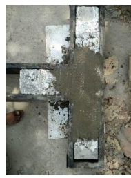
Figure 6: Specimen after rehabilitation
