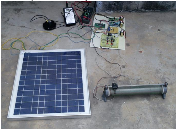
Fig. 5: Hardware Implementation of the system
