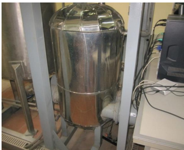
Fig. 3: The Steam Boiler Controlling Water Level.
