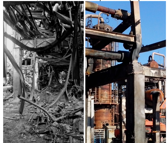
Fig. 3: Deformations after fire obtained by Trimble TX5 laser scanner
