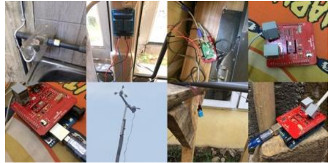
Fig. 6: Implementation of relay and temperature, humidity, wind speed, and light intensity sensors
