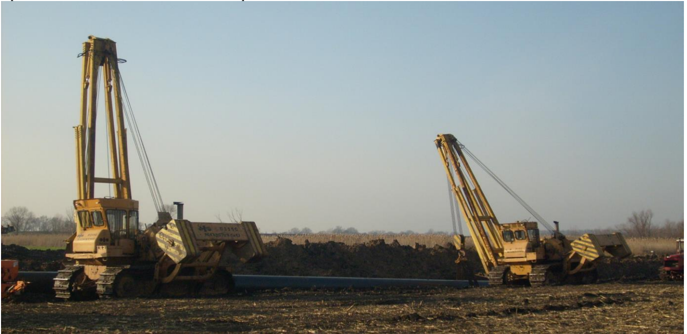
Fig. 1: The process of the main oil pipeline new section installation by the pipe-laying machine D-355
