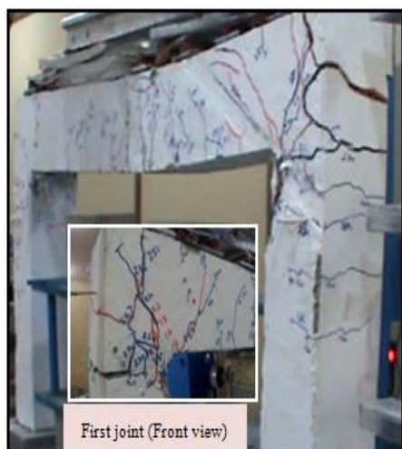
Fig. 8: Crack pattern for frame Fu-Co
