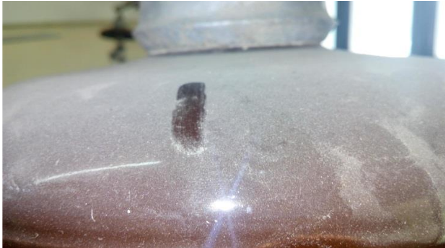
Fig. 12 (A): Uncoated Post Insulator with Formation of Dust Layer.
