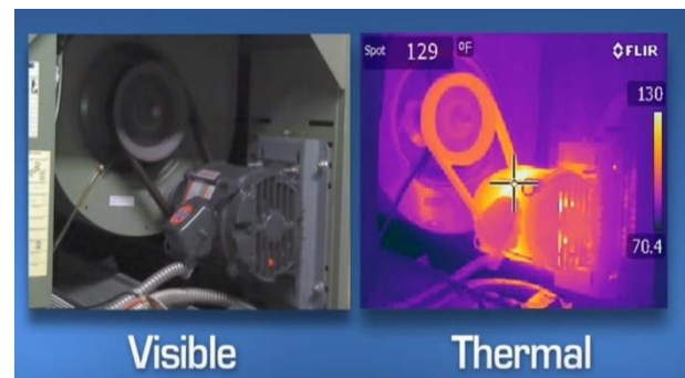
Fig. 1: Thermal Imaging Helps Find/Solve Problems in Process Equipment with Abnormal Heat Flow. (Www.Thermalimagercamera.Com).
